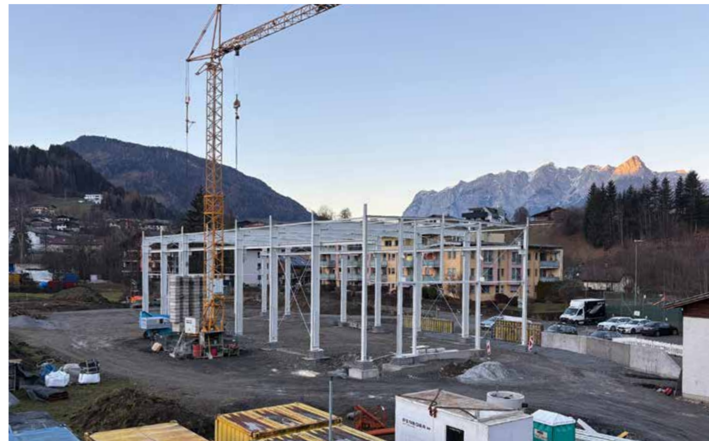
Top: Construction work began at the end of 2025. From the very beginning, great importance was placed on maintaining an open and informative dialogue with local residents Bottom: While the exterior walls were being completed, preparations for the interior fit-out of the hall were already underway in parallel.
